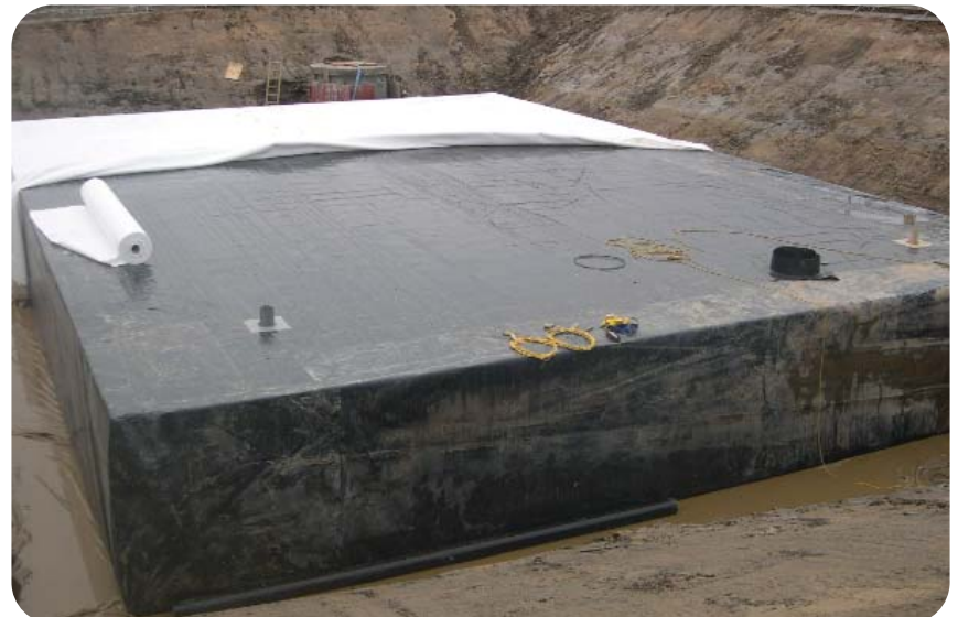
2mts deep tank with 3mts cover
